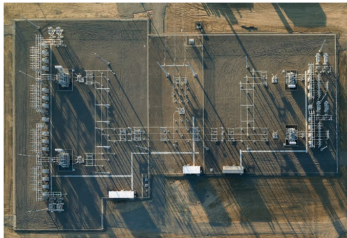
Solar Blue | Stratford, California | 34.5/230kV, 250MVA
