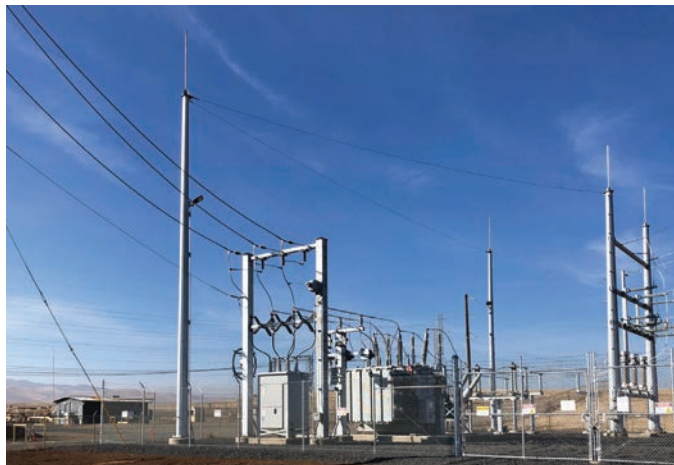
Central 40 | CA | 52.5 MVA, 34.5/115kV
