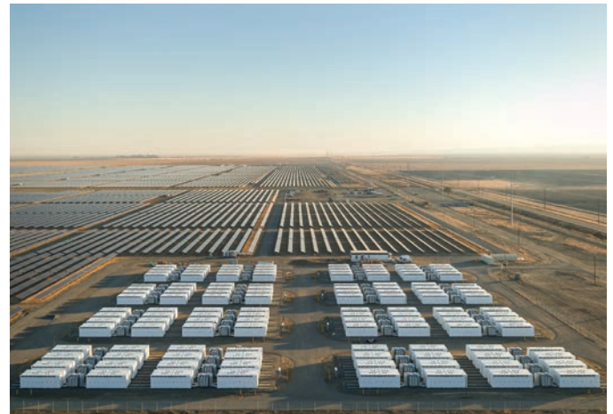
Solar Blue | Stratford, California | 900MWh
