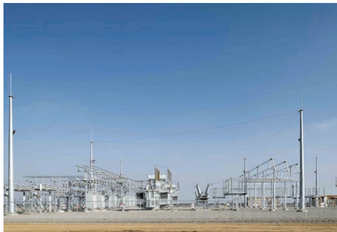
Aquamarine | Stratford, CA | 34.5/230kV and 320MVA
