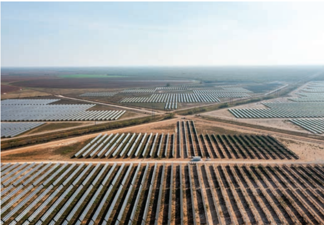
Elara Solar | Pearsall, Texas | 130MW
