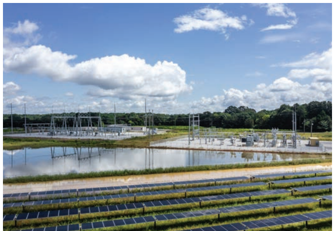
Muscle Shoals Solar | AL | 250MVA, 34.5/161kV
