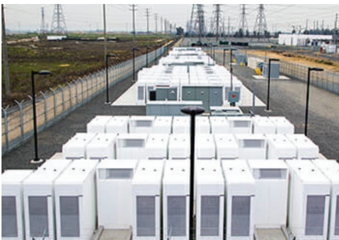
Mira Loma/—Tesla | Ontario, CA | 20MW/80MWh
