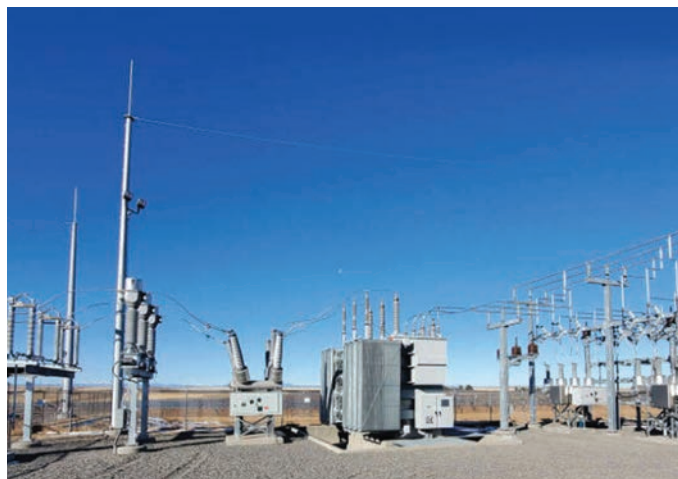
Pioneer Solar | CO | 88.8 MVA, 34.5/115kV
