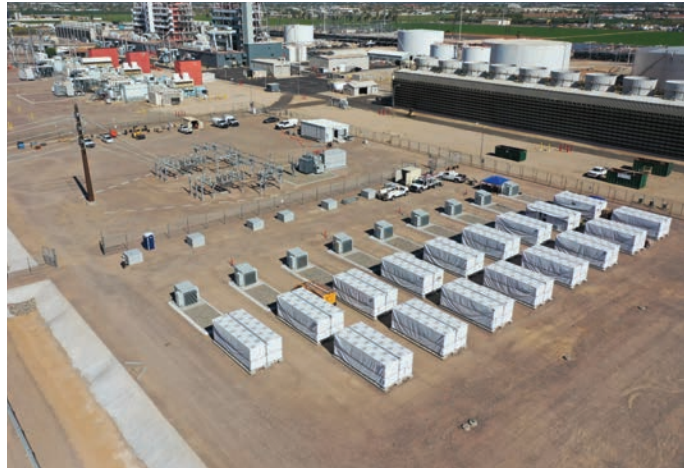
Agua Fria | Glendale, Arizona | 25MW/100MWh
