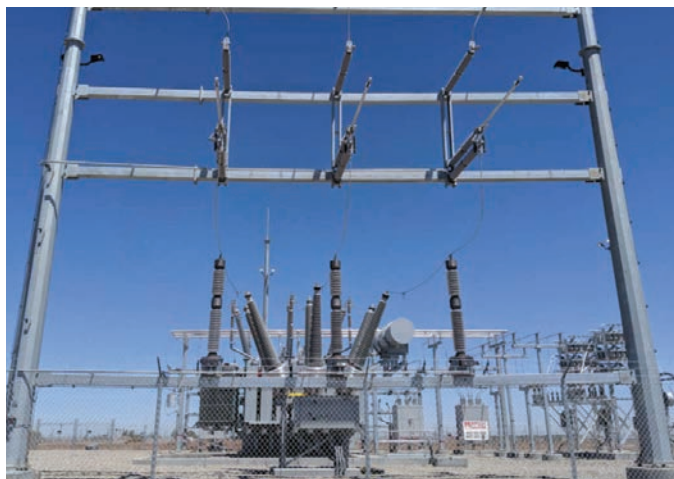
Mount Signal 2 Solar | CA | 165 MVA, 34.5/230kV
