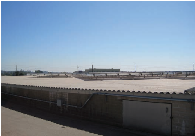
City of Brea, CA | 2MW
