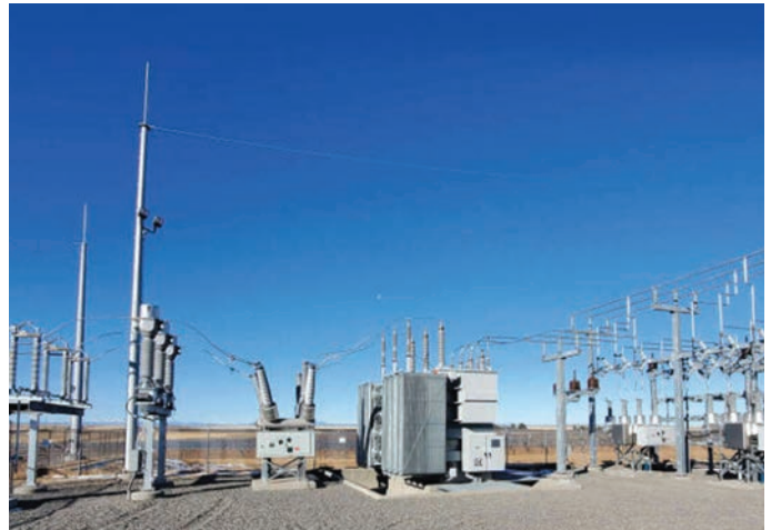
Pioneer Solar | CO | 88.8 MVA, 34.5/115kV
