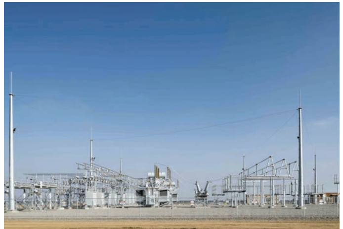
Aquamarine | Stratford, CA | 34.5/230kV and 320MVA
