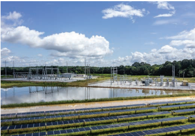
Muscle Shoals Solar | AL | 250MVA, 34.5/161kV
