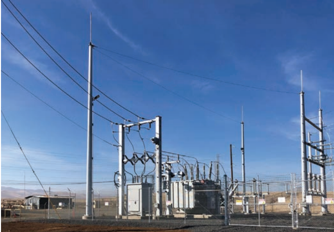
Central 40 | CA | 52.5 MVA, 34.5/115kV
