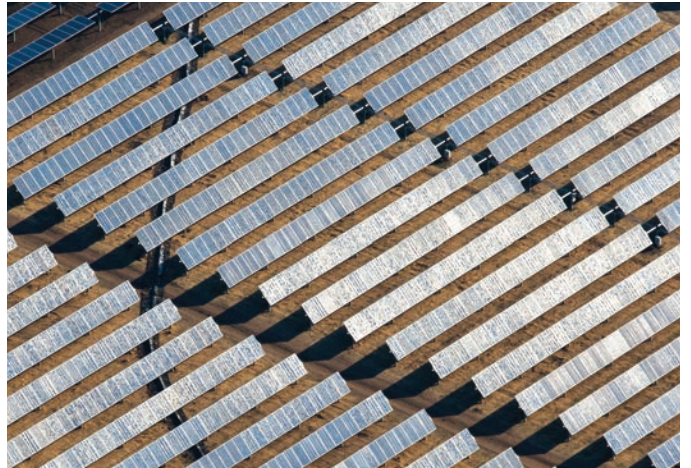
Red Hills Solar Power Plant | Parowan, Utah, 80MW
