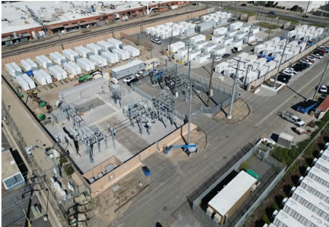
Santa Ana Energy Storage | California | 40MW/160MWh
