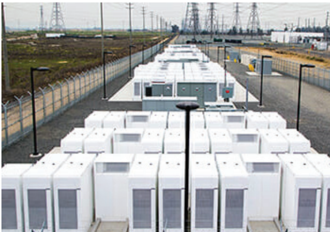
Mira Loma/—Tesla | Ontario, CA | 20MW/80MWh
