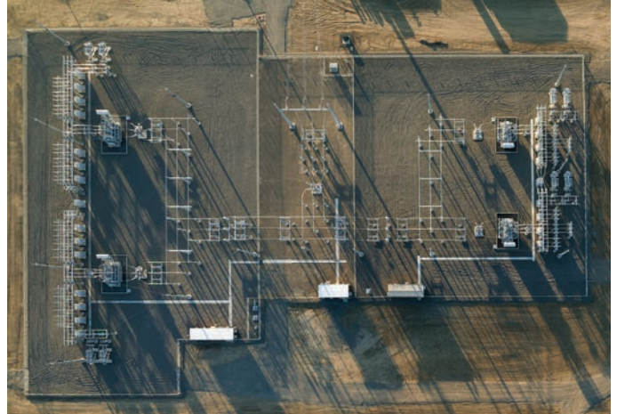
Solar Blue | Stratford, California | 34.5/230kV, 250MVA
