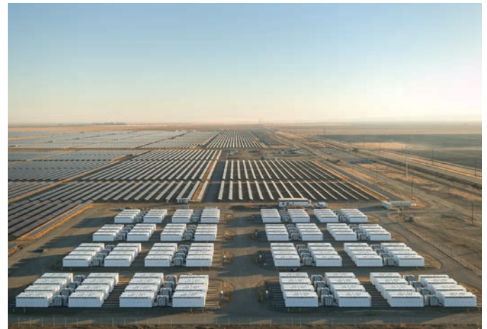
Solar Blue | Stratford, California | 900MWh
