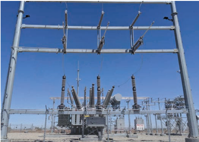
Mount Signal 2 Solar | CA | 165 MVA, 34.5/230kV
