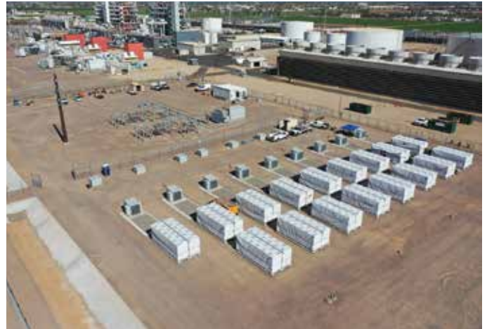
Agua Fria | Glendale, Arizona | 25MW/100MWh
