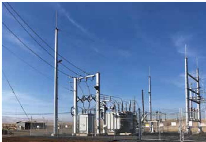
Central 40 | CA | 52.5 MVA, 34.5/115kV
