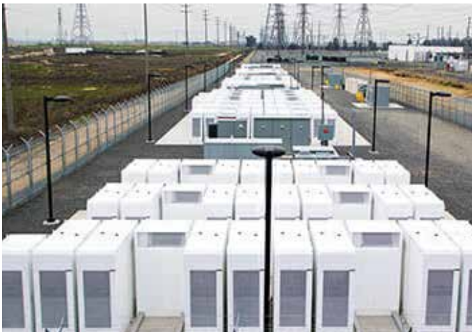
Mira Loma/—Tesla | Ontario, CA | 20MW/80MWh
