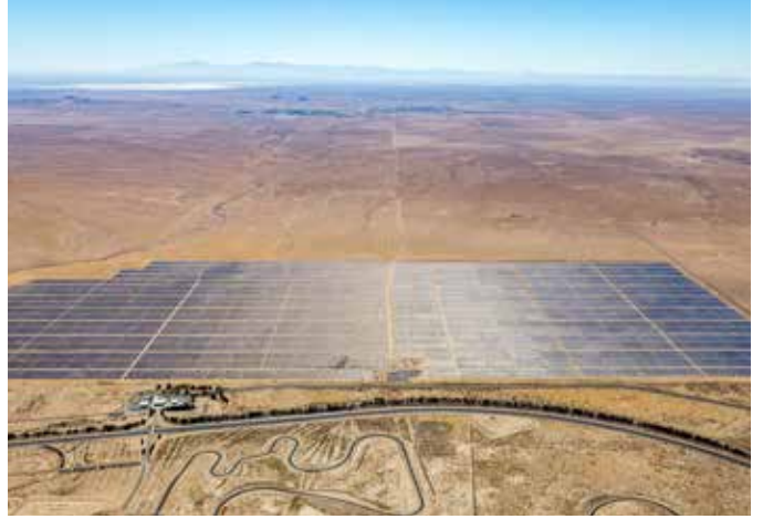
Springbok I and II Solar Plants | Kern County, CA | 258MW
