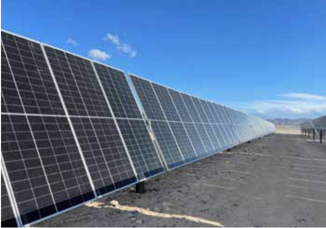
Oberon 1 & 2 | California | 500 MW
