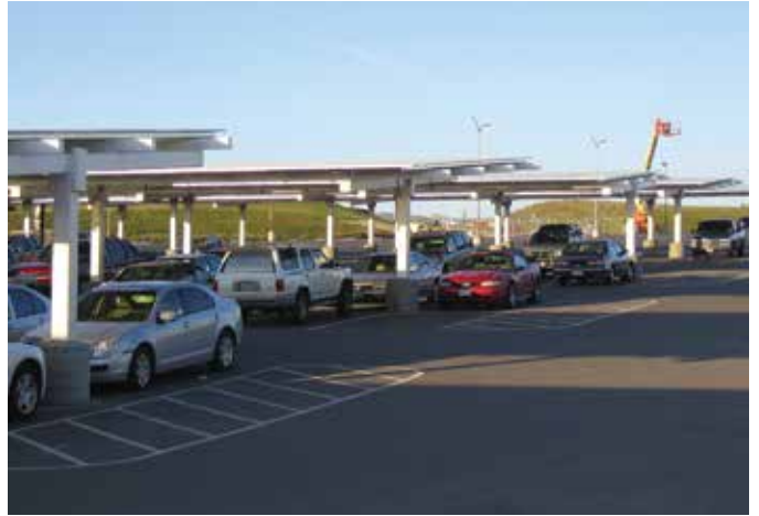
Lancaster Unified School District | 23 schools, CA | 5.5MW
