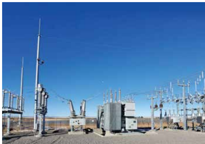
Pioneer Solar | CO | 88.8 MVA, 34.5/115kV
