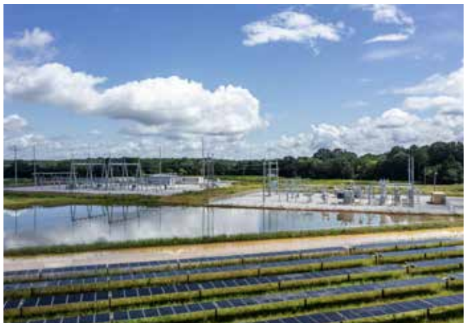
Muscle Shoals Solar | AL | 250MVA, 34.5/161kV
