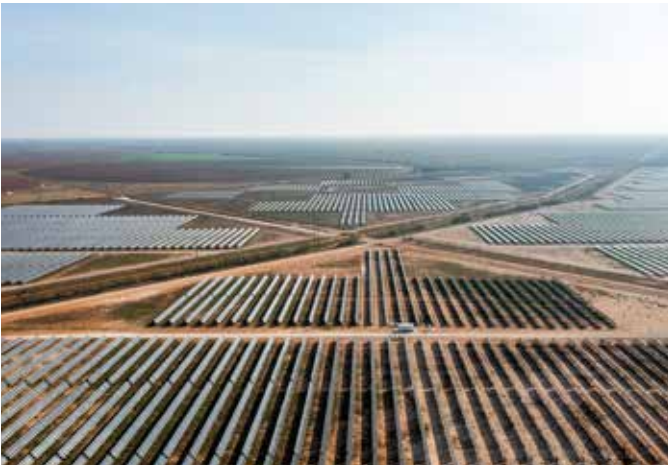
Elara Solar | Pearsall, Texas | 130MW
