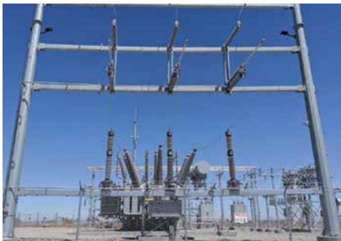
Mount Signal 2 Solar | CA | 165 MVA, 34.5/230kV
