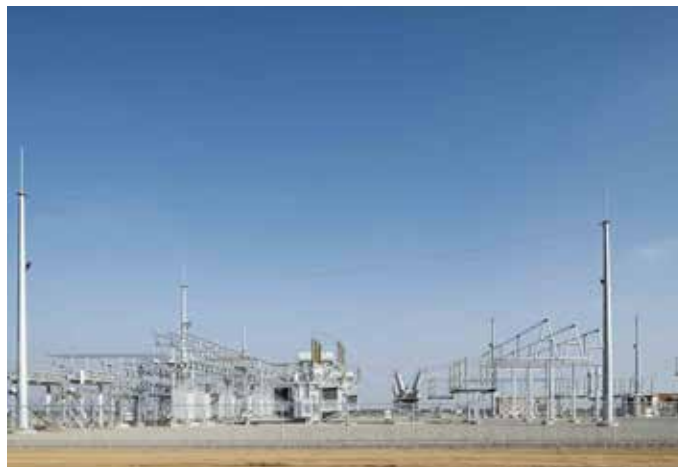
Aquamarine | Stratford, CA | 34.5/230kV and 320MVA
