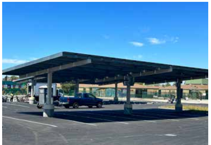
Franklin-McKinley School District, CA | 2.74MW
