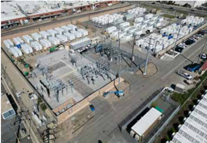
Santa Ana Energy Storage | California | 40MW/160MWh
