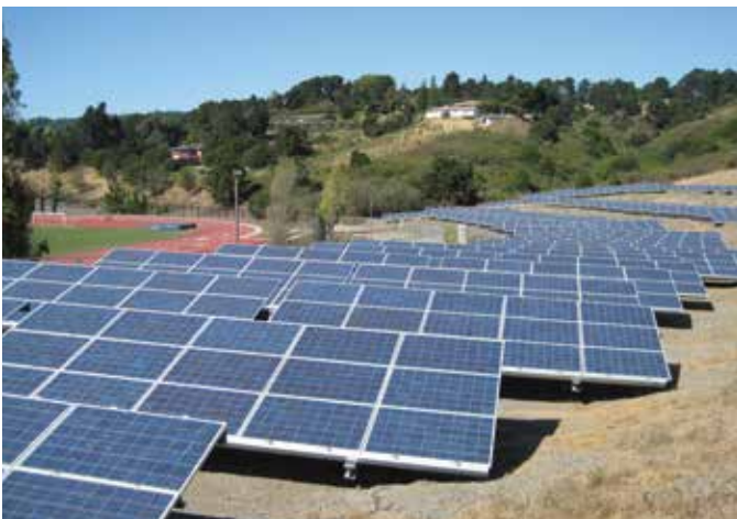
Merritt College, CA | 1.2MW
