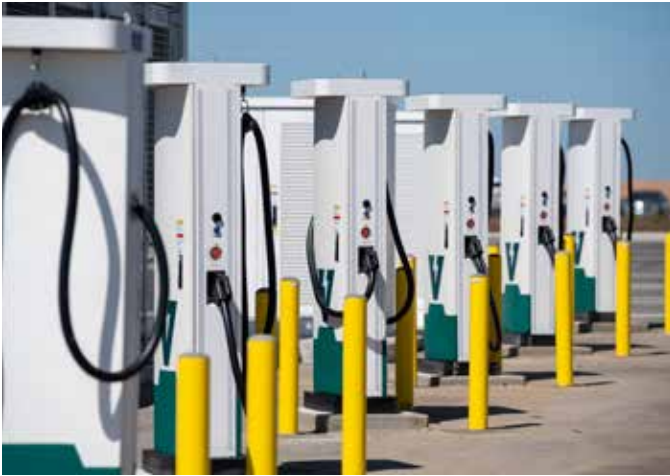
WattEV | Bakersfield, CA | 240-360kW
