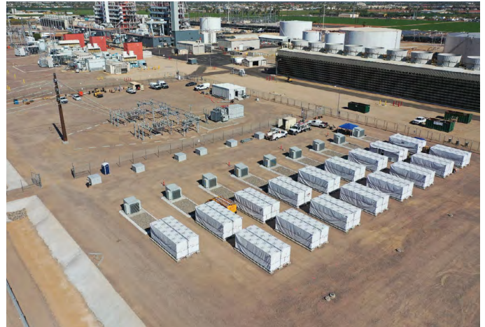
Agua Fria | Glendale, Arizona | 25MW/100MWh
