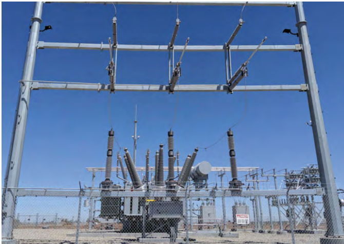
Mount Signal 2 Solar | CA | 165 MVA, 34.5/230kV
