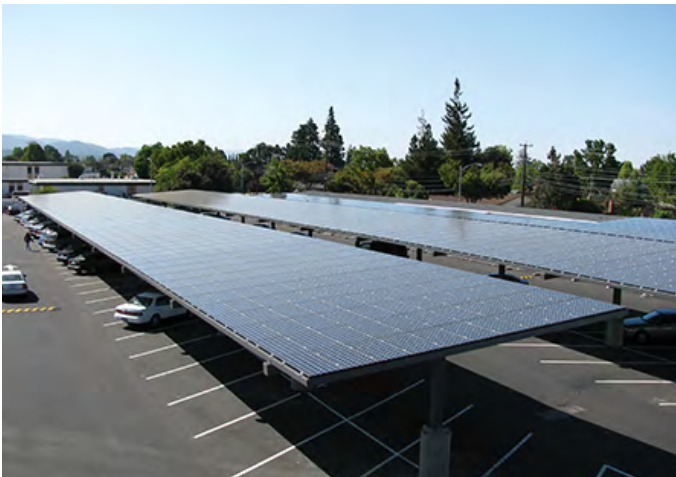
Fremont Union School District | 5 schools, CA | 6.6MW
