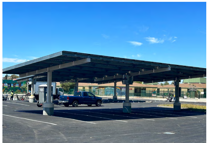
Franklin-McKinley School District, CA | 2.74MW
