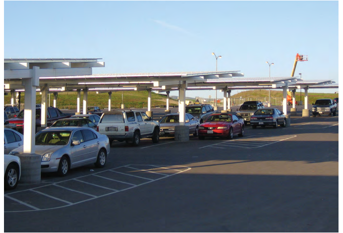
Lancaster Unified School District | 23 schools, CA | 5.5MW
