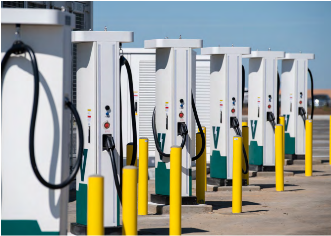
WattEV | Bakersfield, CA | 240-360kW
