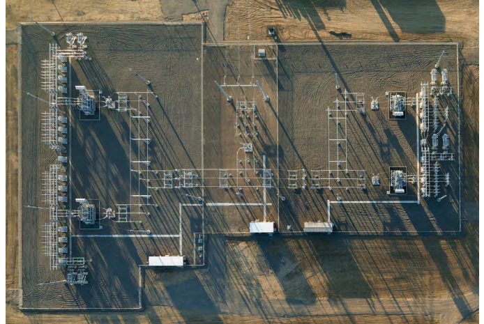
Solar Blue | Stratford, California | 34.5/230kV, 250MVA
