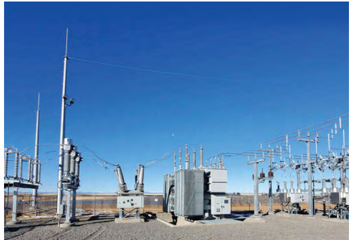
Pioneer Solar | CO | 88.8 MVA, 34.5/115kV
