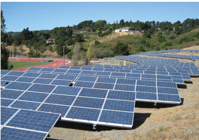
Merritt College, CA | 1.2MW
