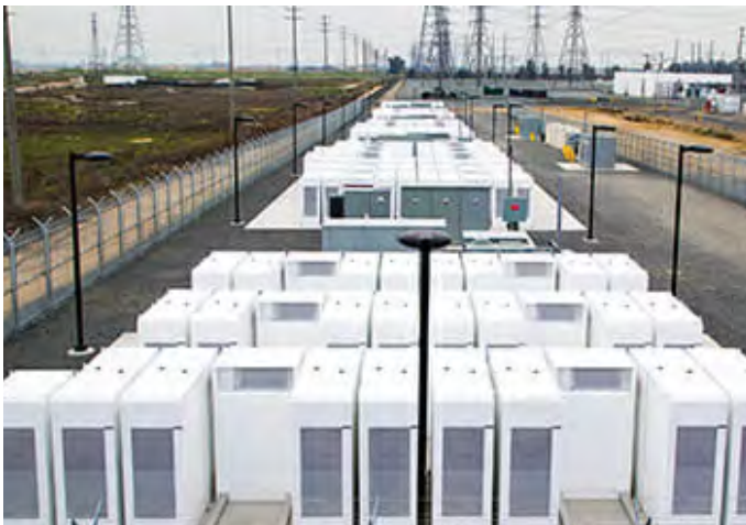
Mira Loma/—Tesla | Ontario, CA | 20MW/80MWh
