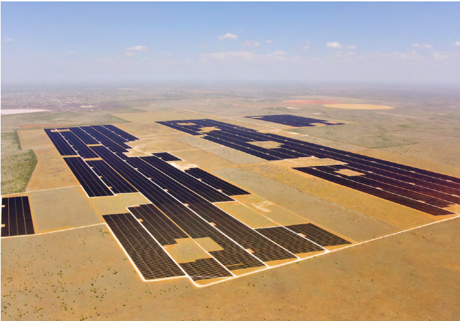
Prospero 1 & 2 | Andrews, Texas | 550MW
