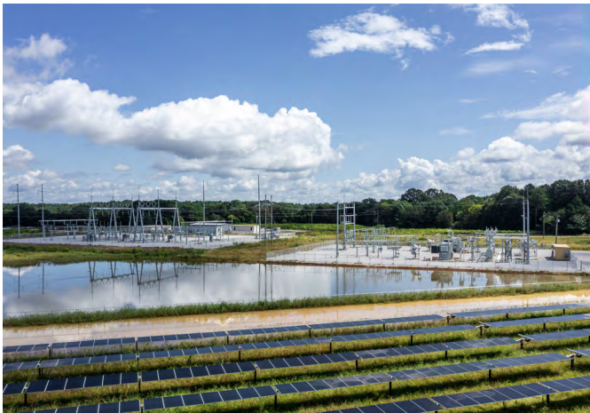
Muscle Shoals Solar | AL | 250MVA, 34.5/161kV
