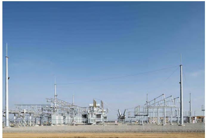
Aquamarine | Stratford, CA | 34.5/230kV and 320MVA
