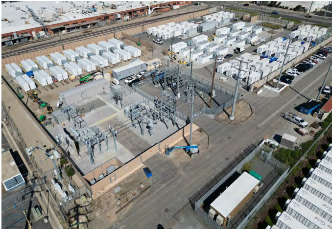
Santa Ana Energy Storage | California | 40MW/160MWh
