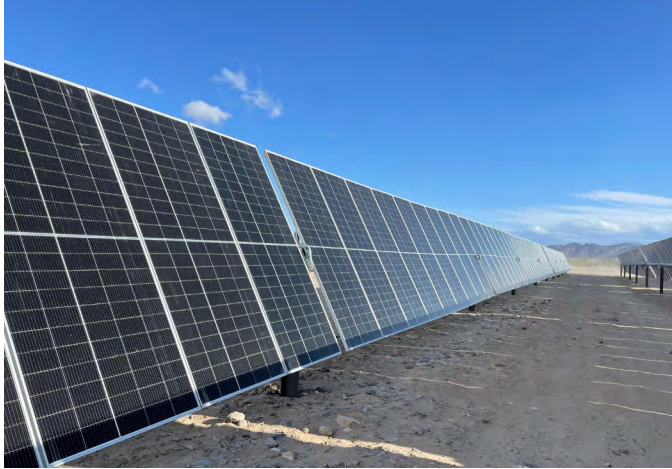
Oberon 1 & 2 | California | 500 MW
