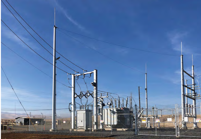
Central 40 | CA | 52.5 MVA, 34.5/115kV
