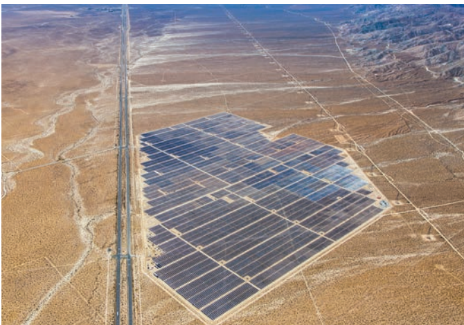
RE Barren Ridge | Kern County, CA | 60MW
