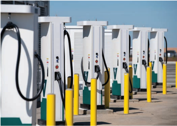
WattEV | Bakersfield, CA | 240-360kW
