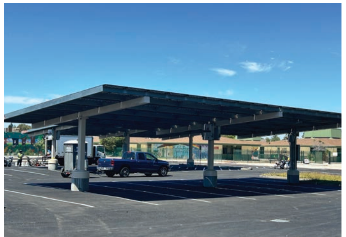
Franklin-McKinley School District, CA | 2.74MW
