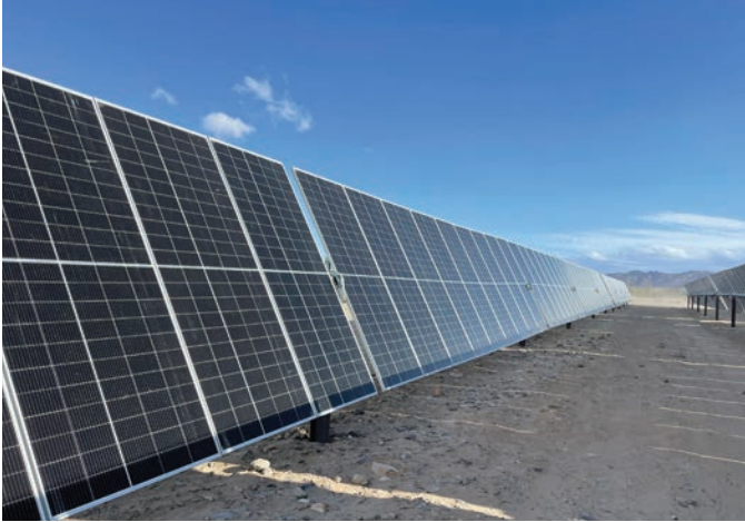
Oberon 1 & 2 | California | 500 MW
