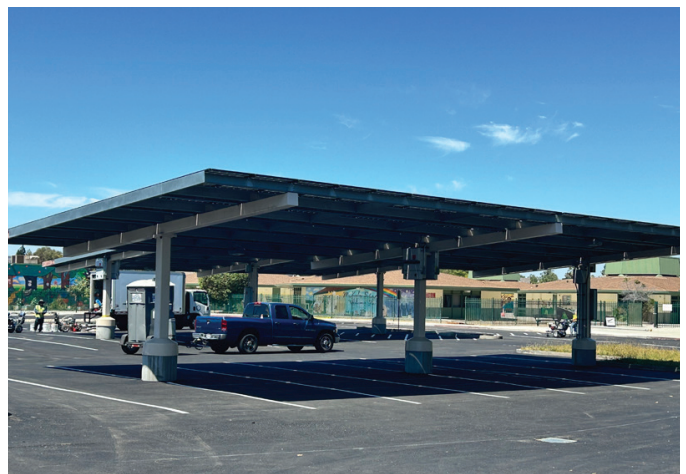
Franklin-McKinley School District | California 2.74 MW Solar
