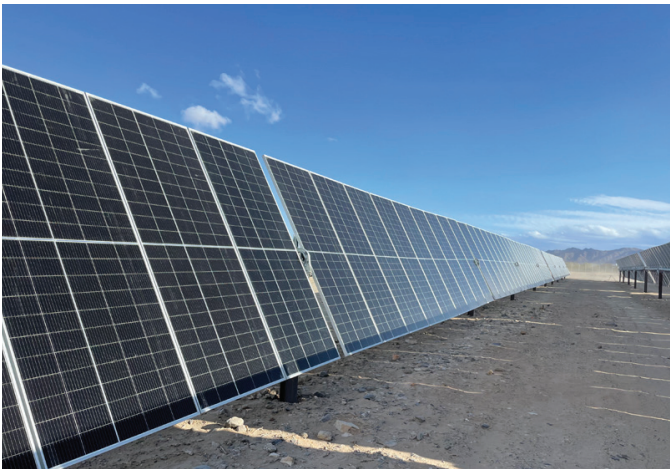
Oberon 1 & 2 | California 500 MW Solar | 250 MWh Energy Storage
