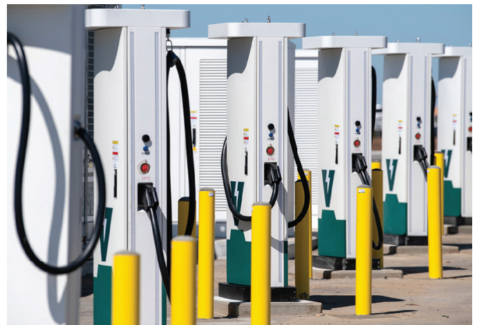
WattEV | Bakersfield, California 3 MWh Energy Storage | 25 MW Solar 240-360 kW EV Charging
