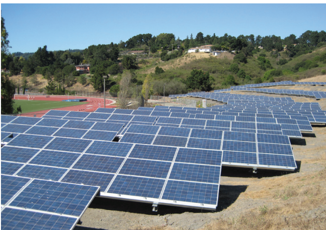
Merritt College | Oakland, California 1.2 MW Solar
