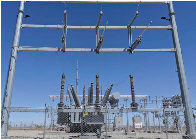
Mount Signal 2 Solar | California 165 MVA, 34.5/230 kV Substation
