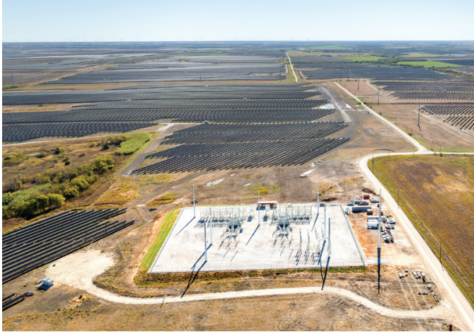
Ash Creek | Abbott, Texas 34.5/345 kV Substation | 408.85 MW Solar
