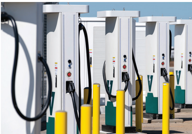
WattEV | Sacramento, California 69 kV Substation | 60 Stalls EV Charging 5.5 MWh Energy Storage | 24.3 MWdc Solar
