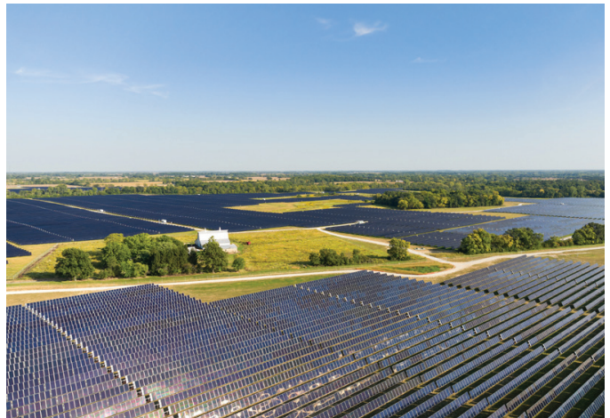
Big Plain | Madison County, Ohio 196 MW Solar | 34.5/138 kV Substation
