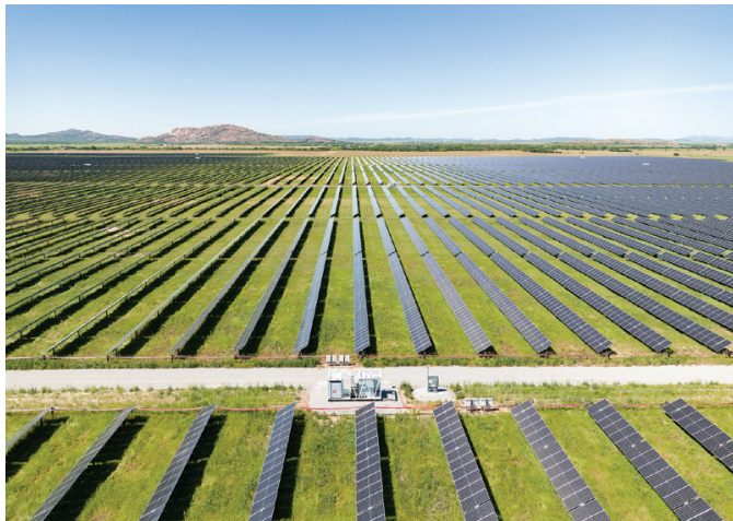
Kiowa County, Oklahoma 34.5/138 kV Substation | 100 MW Solar
