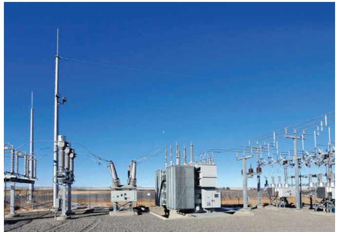
Pioneer Solar | Colorado 88.8 MVA, 34.5/115 kV Substation
