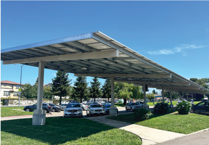
Pinole Valley High School | California 418 kW Solar
