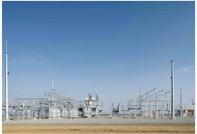
Aquamarine | Stratford, California 320 MVA, 34.5/230 kV Substation
