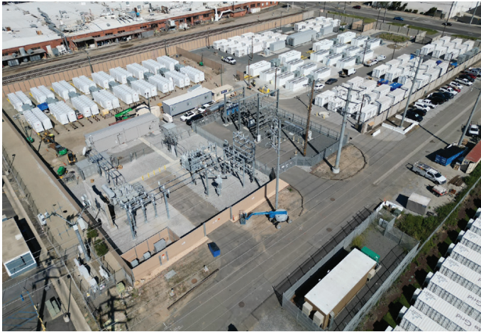
Santa Ana Energy Storage | California 40 MW/160 MWh Energy Storage
