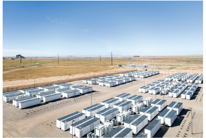
San Juan | Kirtland, New Mexico 400 MWh Energy Storage | 200 MW Solar
