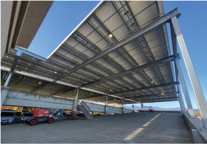
County of Shasta, California | 16 Sites 2.5 MW Solar
