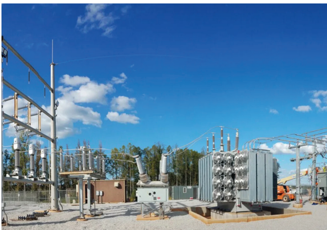
Chambers County, Alabama 34.5/115 kV, 90 MVA Substation 72 MW Solar
