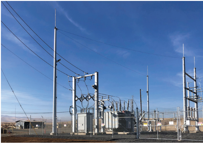
Central 40 | California 52.5 MVA, 34.5/115 kV Substation
