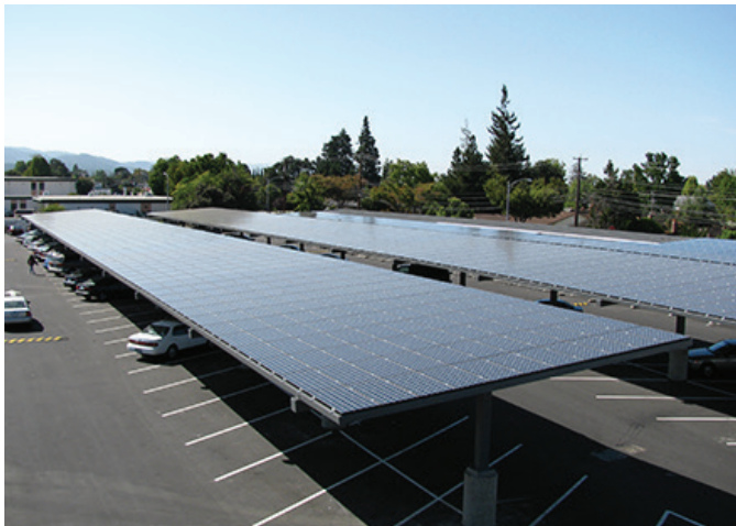
Fremont Union School District | California 6.6 MW Solar | 5 schools
