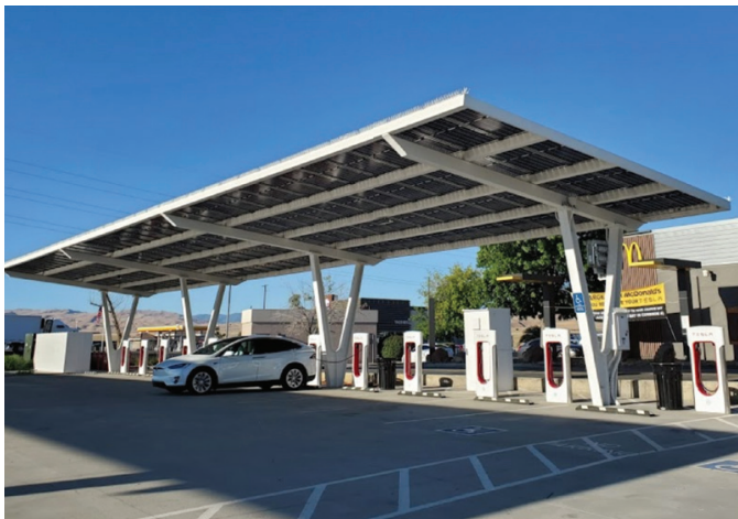
Tesla Firebaugh | Firebaugh, California 56 Stalls EV Charging
