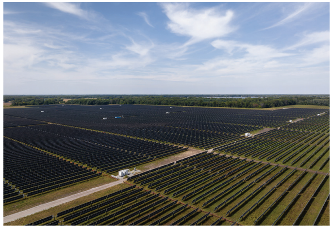
Mammoth North | Monterey, Indiana 400 MW Solar
