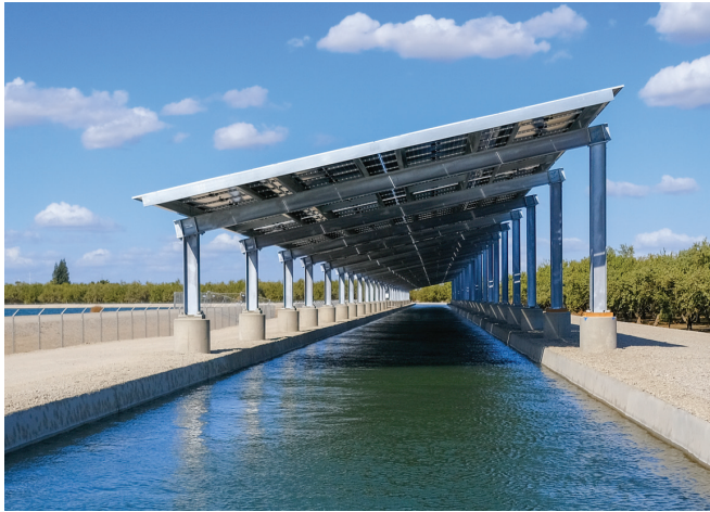
Project Nexus | Stanislaus County, California 1.6 MW Solar | 800 kWh Energy Storage
