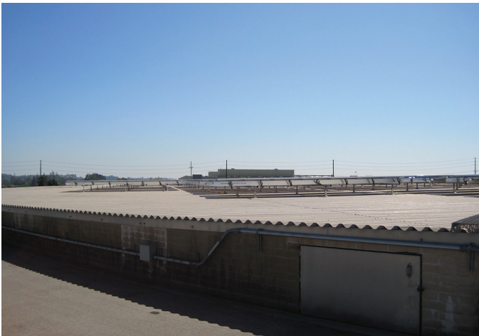
City of Brea, California | 2 MW Solar
