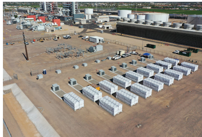
Agua Fria | Glendale, Arizona 25 MW/100 MWh Energy Storage
