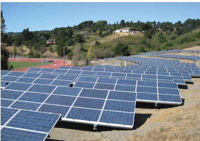
Merritt College | Oakland, California 1.2 MW Solar
