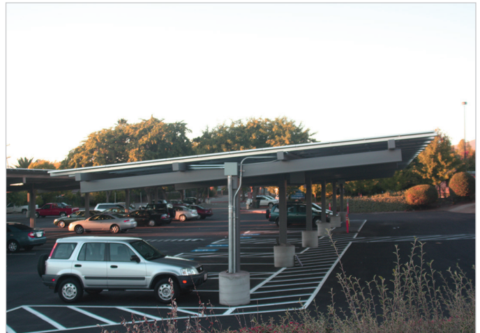
Milpitas Unified School District | California 3.4 MW Solar | 14 schools
