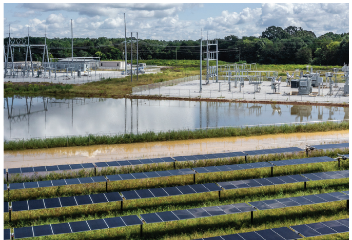
Muscle Shoals | Colbert County, Alabama 227 MW Solar | 34.5/161 kV Substation
