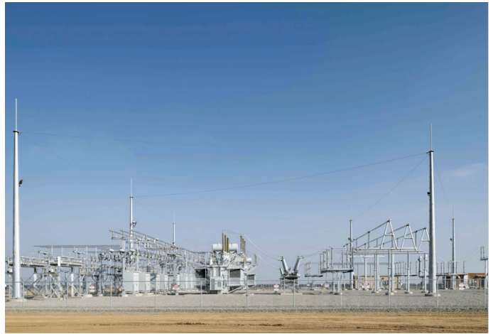
Aquamarine | Stratford, California 320 MVA, 34.5/230 kV Substation
