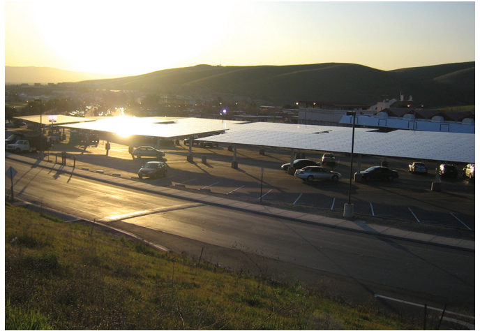
Las Positas Community College Chabot, California | 2.2 MW Solar
