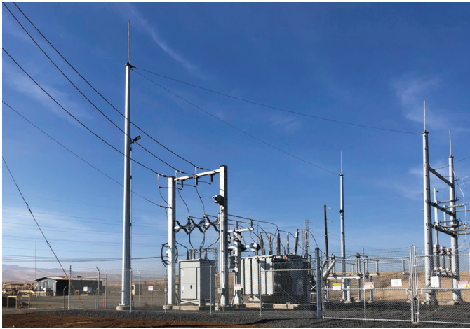
Central 40 | California 52.5 MVA, 34.5/115 kV Substation
