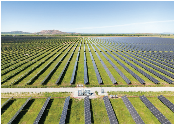
Kiowa County, Oklahoma 34.5/138 kV Substation | 100 MW Solar
