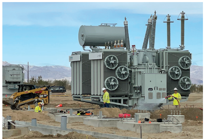
Victory Pass & Arica | Desert Center, California 34.5/230 kV, 514 MVA Substation 463 MW Solar | 186 MWh Energy Storage
