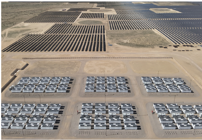
Franklin | Rogerson, Idaho 240 MWh Energy Storage | 100 MW Solar
