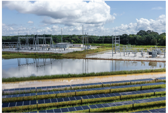
Muscle Shoals | Colbert County, Alabama 34.5/161 kV Substation | 227 MW Solar
