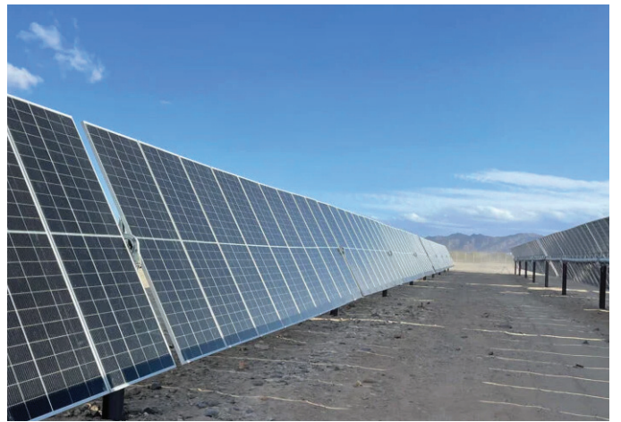
Oberon 1 & 2 | California 250 MWh Energy Storage | 500 MW Solar
