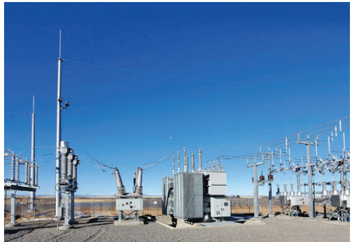
Pioneer Solar | Colorado 88.8 MVA, 34.5/115 kV Substation
