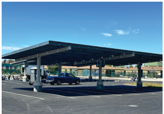
Franklin-McKinley School District | California 2.74 MW Solar
