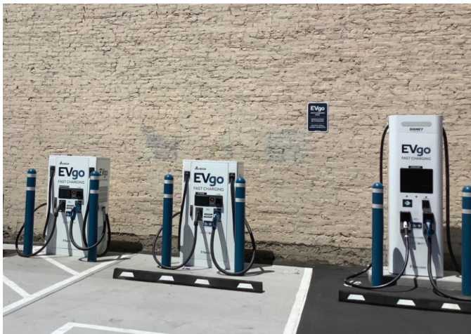
EVgo Pacific Ave | San Francisco, California 24 Stalls EV Charging
