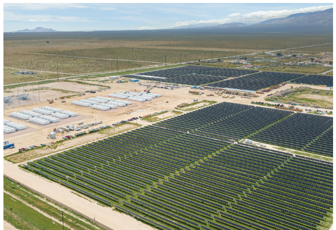
Eland | California City, California 200 MW Solar
