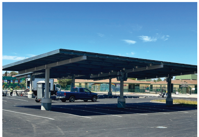
Franklin-McKinley School District | California 2.74 MW Solar
