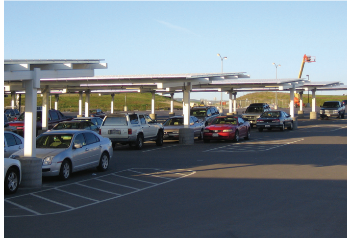
Lancaster Unified School District | California 5.5 MW Solar | 23 schools
