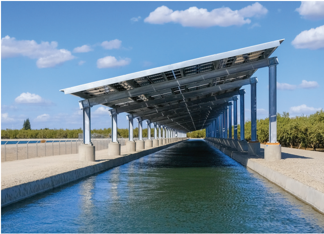
Project Nexus | Stanislaus County, California 1.6 MW Solar | 800 kWh Energy Storage
