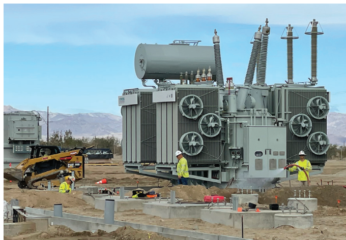
Victory Pass & Arica | Desert Center, California 34.5/230 kV, 514 MVA Substation 463 MW Solar | 186 MWh Energy Storage
