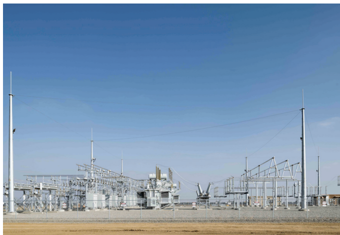
Aquamarine | Stratford, California 320 MVA, 34.5/230 kV Substation
