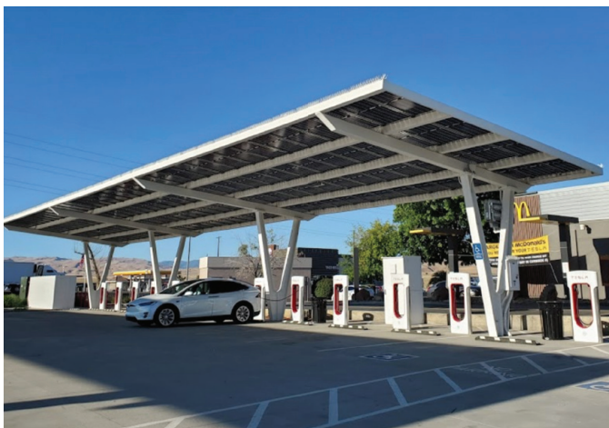
Tesla Firebaugh | Firebaugh, California 56 Stalls EV Charging
