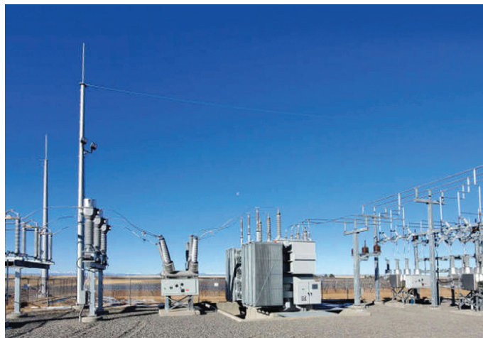
Pioneer Solar | Colorado 88.8 MVA, 34.5/115 kV Substation
