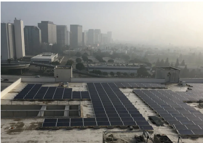
U.S. Veterans Administration Hospital Florida and California | 5.7 MW Solar
