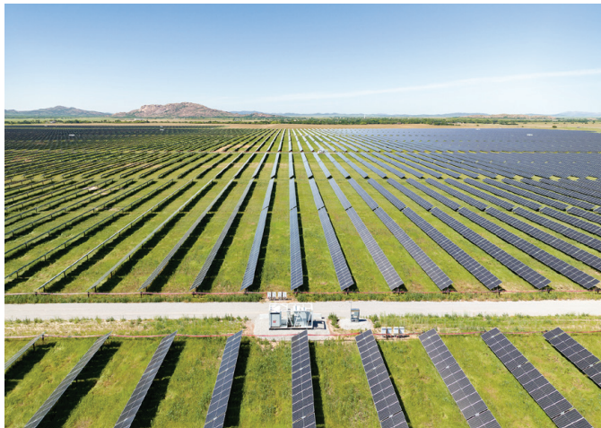
Kiowa County, Oklahoma 34.5/138 kV Substation | 100 MW Solar
