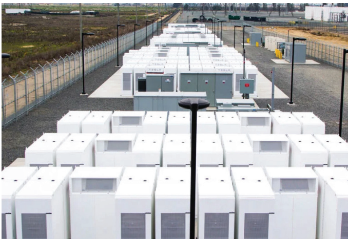
Mira Loma/Tesla | Ontario, California 20 MW/80 MWh Energy Storage
