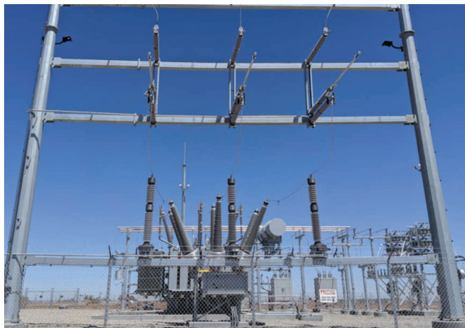
Mount Signal 2 Solar | California 165 MVA, 34.5/230 kV Substation
