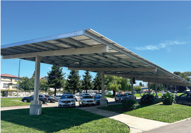
Pinole Valley High School | California 418 kW Solar
