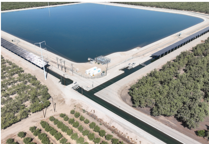
Project Nexus | Stanislaus County, California 800 kWh Energy Storage | 1.6 MW Solar
