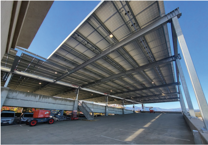
County of Shasta, California | 16 Sites 2.5 MW Solar
