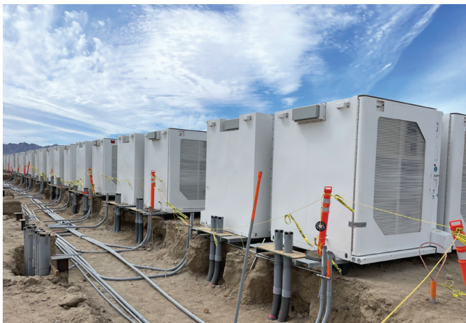
Victory Pass & Arica | Desert Center, California 186 MWh Energy Storage | 463 MW Solar
