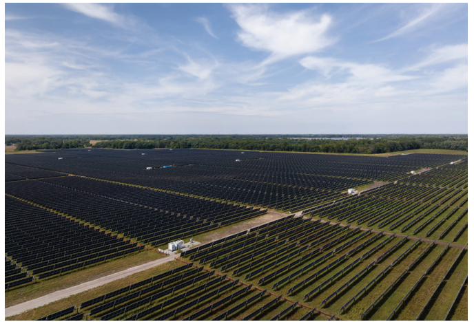
Mammoth North | Monterey, Indiana 400 MW Solar
