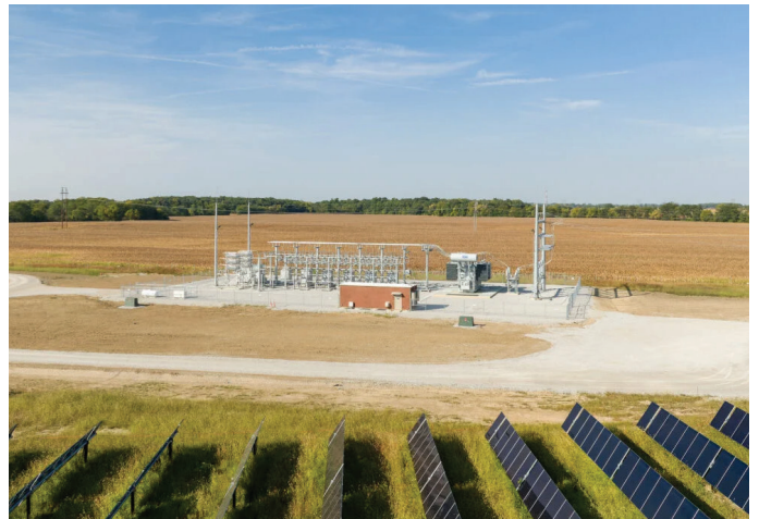
Big Plain | Madison County, Ohio 34.5/138 kV Substation | 196 MW Solar
