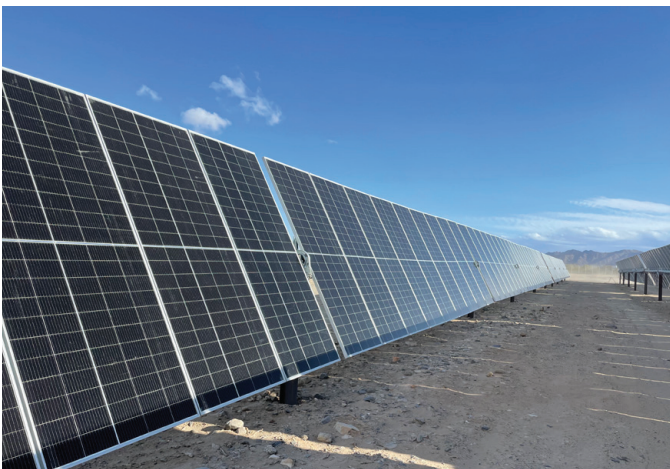
Oberon 1 & 2 | California 500 MW Solar | 250 MWh Energy Storage
