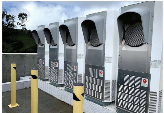
Tesla City Center | San Francisco, California 40 Stalls EV Charging
