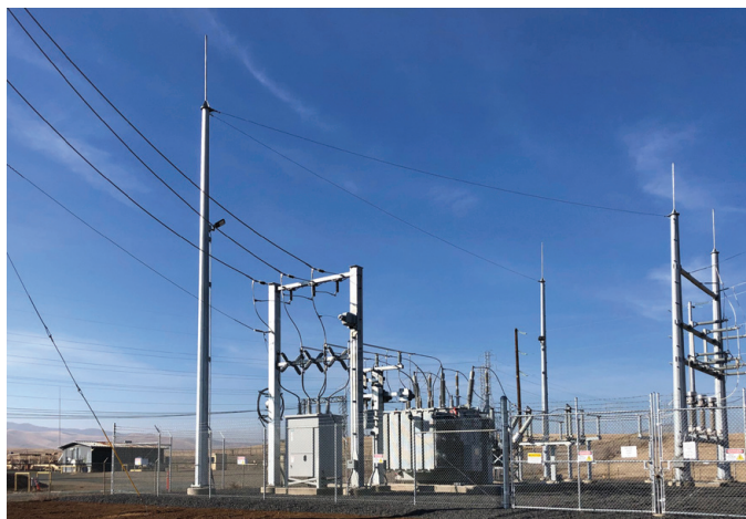
Central 40 | California 52.5 MVA, 34.5/115 kV Substation
