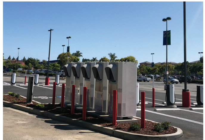
Tesla Gateway 101 | East Palo Alto, California 20 Stalls EV Charging
