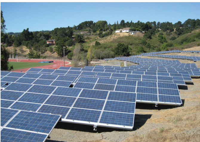
Merritt College | Oakland, California 1.2 MW Solar
